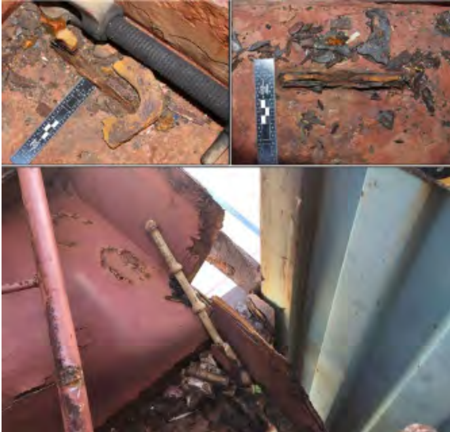
Figure 1. Thinned, heavily wasted and failed lashing eyes (top) and wasted and failed container support structure (bottom)
